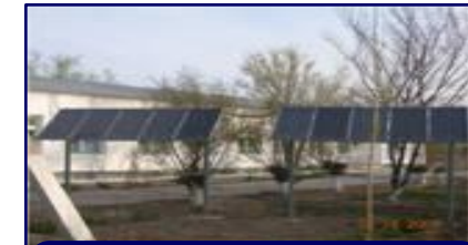
Solar PV system
