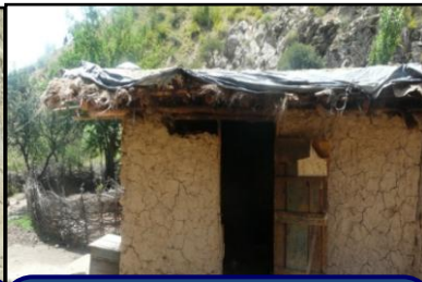
Poor insulation resulting in high heat losses
