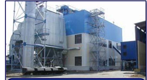
Vileyka biomass cogeneration plant
