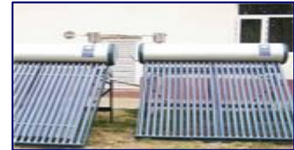
Solar Water Heating system in rural clinic: 4 m 2 , 250l, $2300
