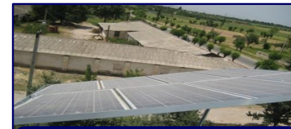
PV system on the roof of hospital
